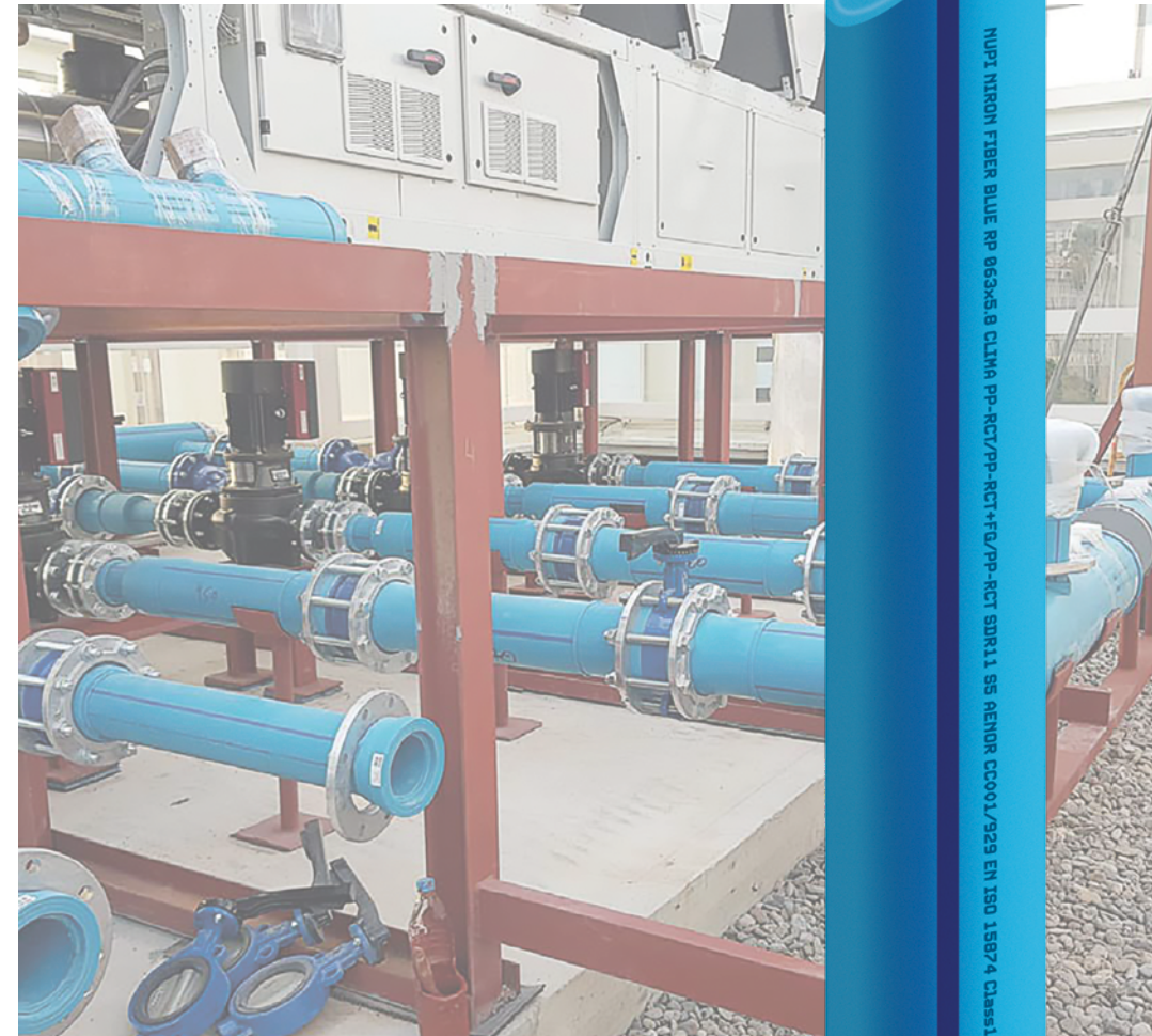
Image provided by Instalaciones Arumani Iberica. HVAC installation CPD BSC MareNostrum BCN.
